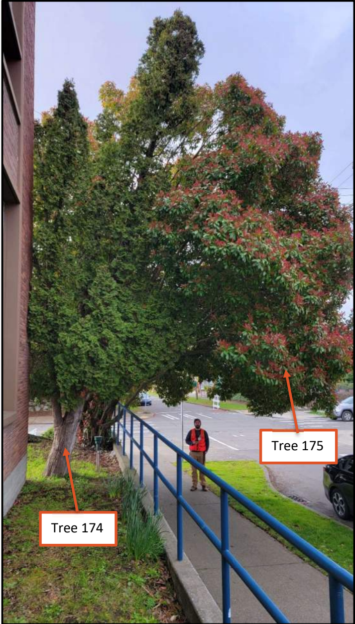
Photo 4. Trees 174 and 175 are growing adjacent to and are dependent on the retaining wall along 38 th Ave S. (April 2023)
